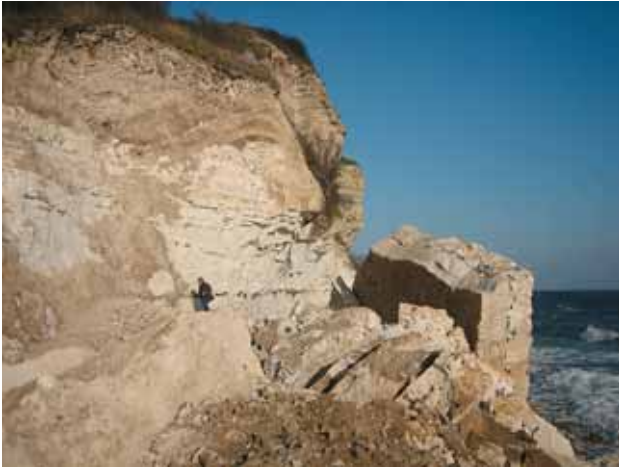
Fig. 6. The cliff collapse at Knøsen, which occurred in November 2011. The weight of fill deposited on top of the section added to the load of the overhang.
